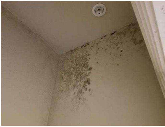
Photo of microbial growth along interior wall of a closet primarily due to vapor pressure diffusion from attic into plenum space above.
