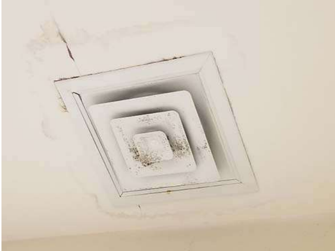
Photo of moisture/condensation stains around supply diffuser due to lack of properly installed insulation.
