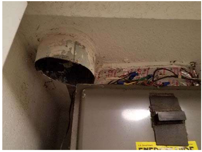
Photo of outdoor air duct stubbed into apartment AHU plenum closet. Not ideal but would be better to duct down to return air opening of AHU and provide volume damper for control.
