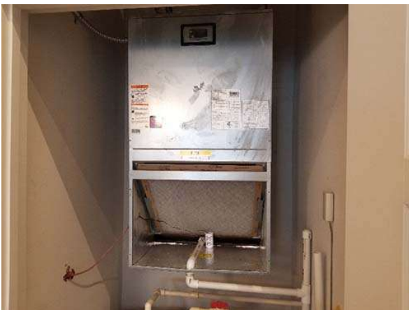
Typical residential type AHUs may not be suitable for high efficiency MERV-13 or above filters. Verify the AHU performance including ductwork layout to determine if such filters are suitable for its intended application.
