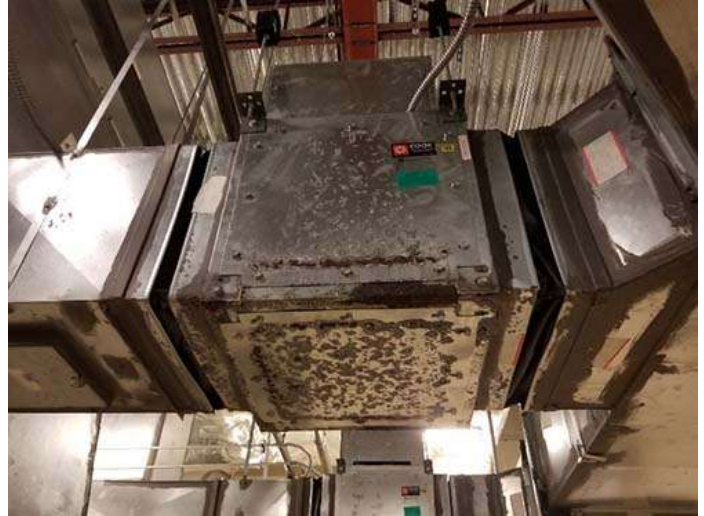
Example of excessive non-conditioned outdoor air effects into an outdoor air fan/duct system causing deterioration and corrosion of surrounding equipment and materials
